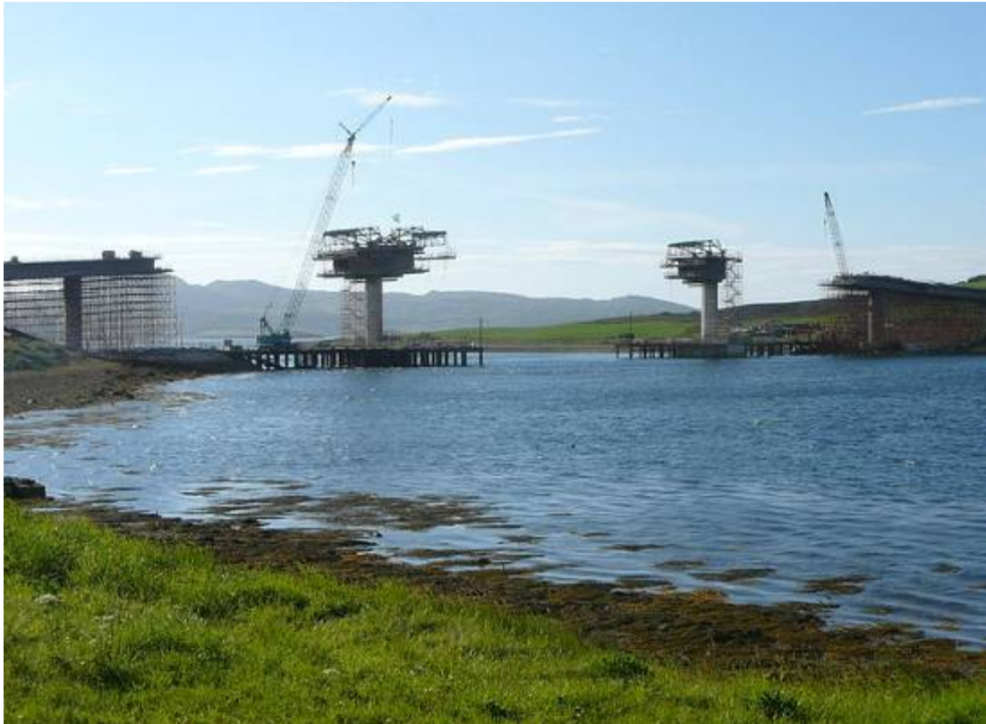
Figure 2.4. New bridge in the second narrow area in Mulroy Bay. Copyright Colin Park and licensed for reuse under this Creative Commons Licence
