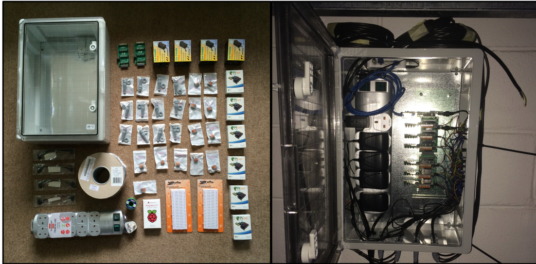
Figure 2.18. Main control box pre and post assembly.
