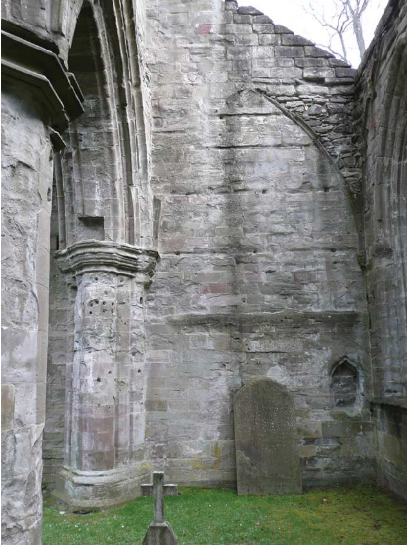
Fig 30. Dunkeld cathedral: east wall of the south nave aisle. The horizontal chases in the wall are perhaps for the fixings of an altar retable; a piscina is seen to the right
