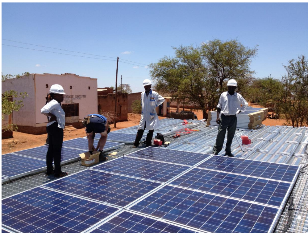
Figure 7. PV system on canopy where local engineers were trained as the project installation progressed and systems were commissioned.
