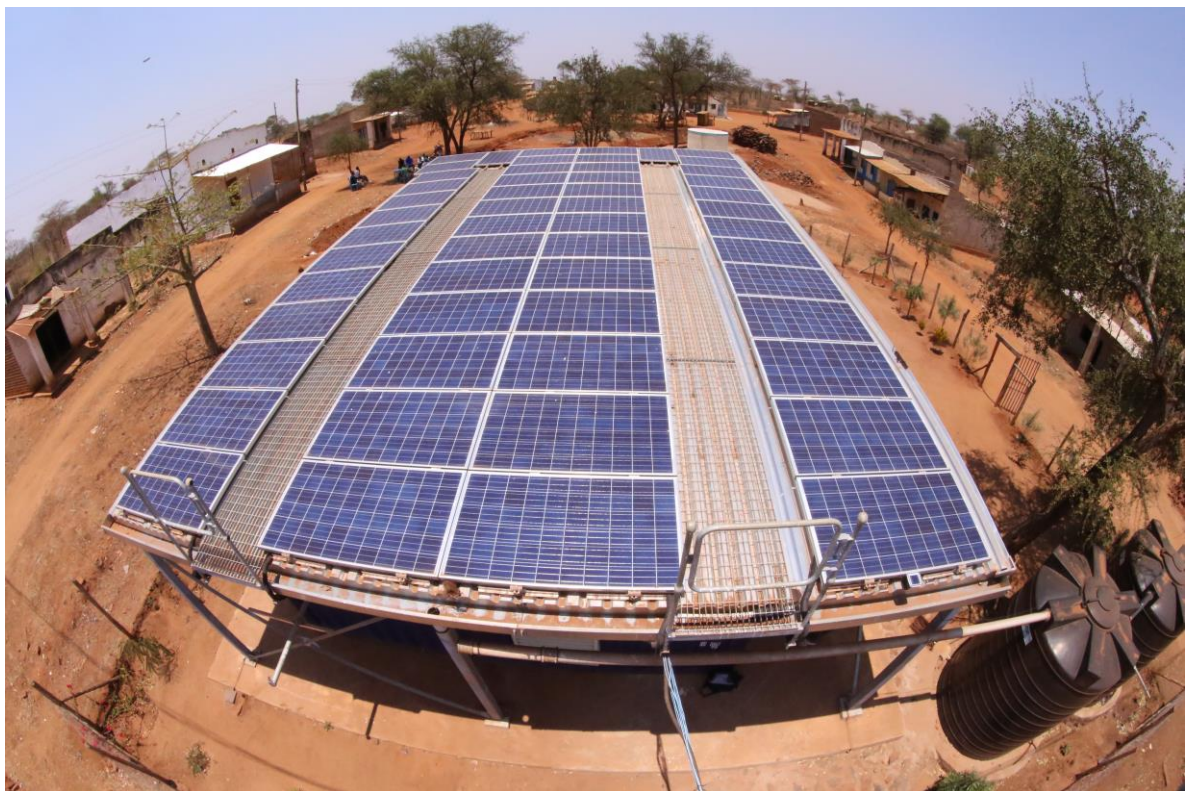
Figure 2. PV system in Kitonyoni trading centre where the modules were installed on a canopy that provides shading for the community as well as harvesting rainwater ( 2 \times 10,000 l storage tanks, front right of image).
