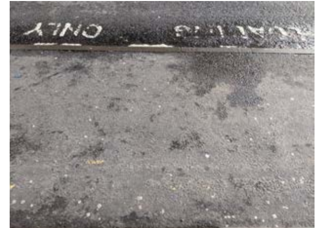
Consider priority drop off stopping for disabled people outside the travel hub. Several areas around the station have paving contrast issues.
