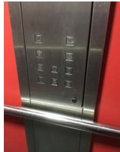
Lift controls are hard to see and understand.
