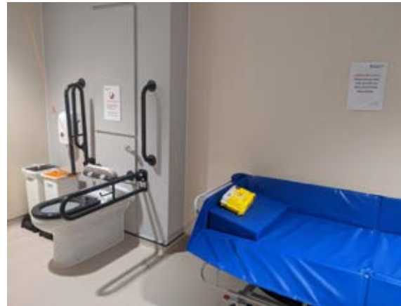
The Changing Places facility in the Bellfield is most welcome but could be better signed.
