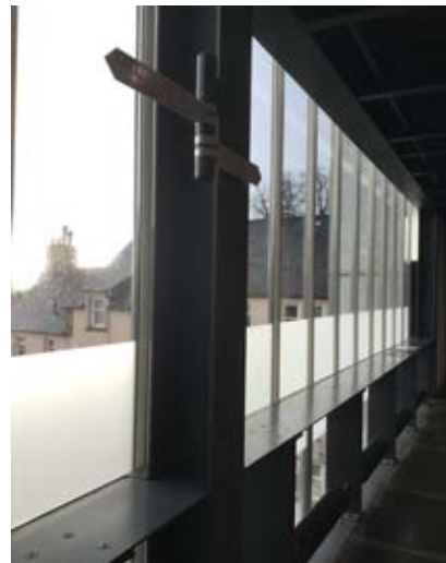
Some signage is poorly located.
