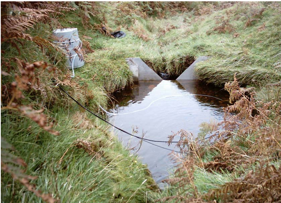
Figure 13: The Ochil Hills 90° thin plate weir, pictured looking a) upstream and b) downstream
